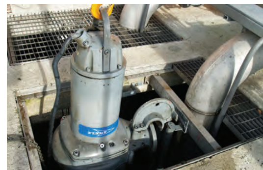
3000 Series Pump Installed
