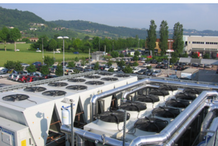
Dry Cooling System, Montecchio, Italy
