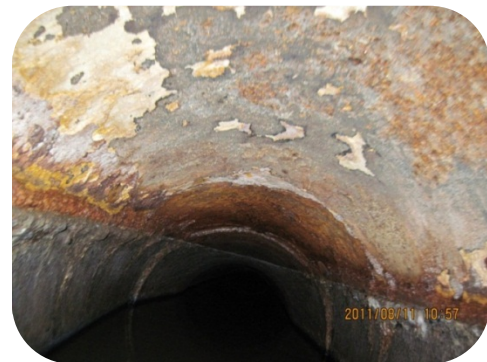
Figure 2.1 – DIP Deterioration Due to Hydrogen Sulfide Corrosion
