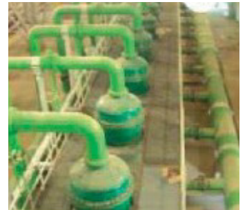
Desalination plant (Beni Saf, Algeria)
