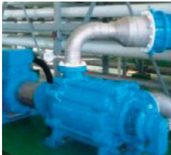
Tertiary treatment (Benidorm, Spain)
