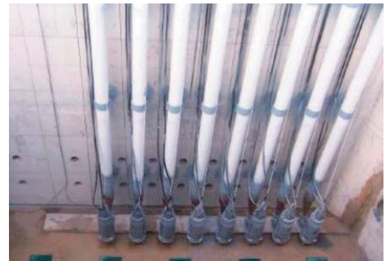
The arguments of Xylem Iberia convinced all parties (contractor, engineering company, technical assistance and end user) and, finally, 8 Flygt submersible pumps (7 +1, with space for another pump), model CP-3240.865 HT 375 kW, were installed to pump the 6,405 m 3 /h of seawater to the desalination plant through a pipe of 1,200 mm diameter and 322 m length.
