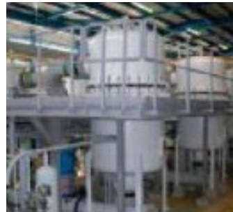
Desalination plant (Fujairah, UAE)
