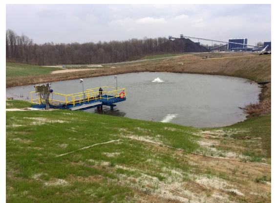
Goulds Water Technology vertical turbine with automated controls on a Xylem-designed custom platform with catwalk supplying water to the preparation plant for washing coal.
