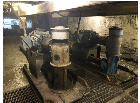
Seven-stage Goulds Water Technology short set vertical turbine pumps – with 90-degree right angle drives and C-face, high-efficiency motors – fit perfectly into the limited space. This reduced both the installed height and the need for an extra five to seven feet of vertical clearance that standard vertical hollow-shaft motors require.
