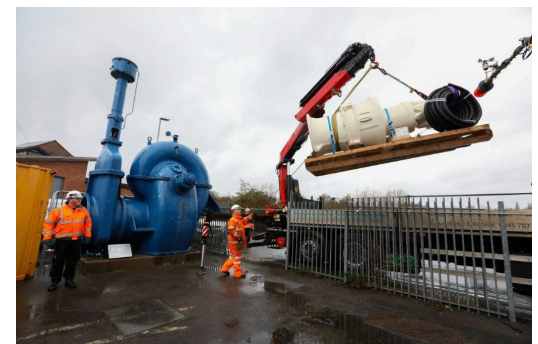
Figure 2. The old and new 'snail pump' from 1963 with its 2021 equivalent about to be installed in the Gloucester Docks on the 7th December 2021.
