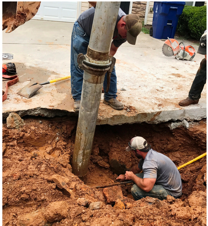
The city utility team uses pressure monitoring and data analytics to identify underground leaks that aren’t visible above ground.
