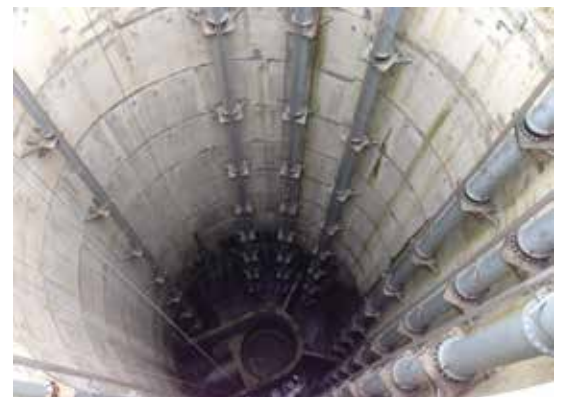
Flygt pumps in a 200' deep wet well
