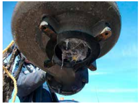
Existing pump lifted for service to remove a fibrous clog
