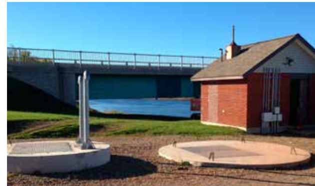
City of Bathurst Lift Station No. 1
