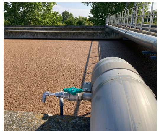
From a mobile unit at the top of the basin, cleaning agent is injected into the main air supply pipe and evenly dispersed to the diffusers with the blower air.
