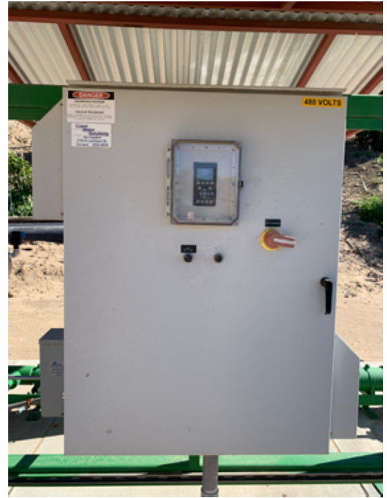
The Aquavar IPC is housed in an optional NEMA 3R steel enclosure featuring thermostatically controlled ventilation fans.
