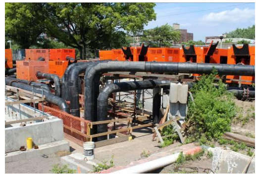
Fifteen Critically Silenced Dri-Prime DPC300 pumps bypassed the plant's flow during a 10-year storm event.
