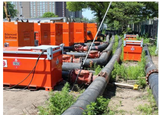
Auxiliary 500-gallon fuel cells connected to the primary pumps.
