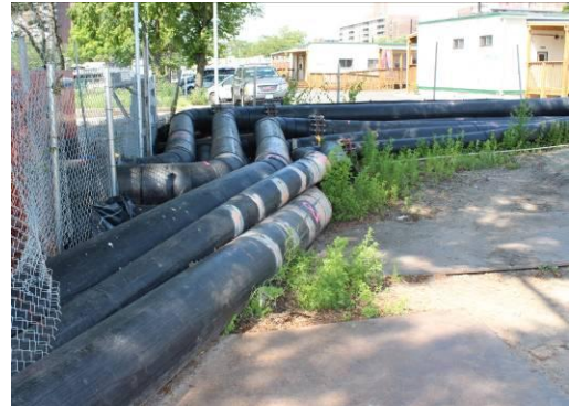
Pipe led the product to the discharge point, a high-level manhole over 500 feet away.
