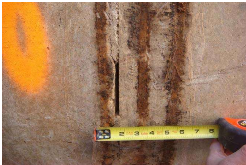
Figure 1 - Poor PCCP Joint Mortar
