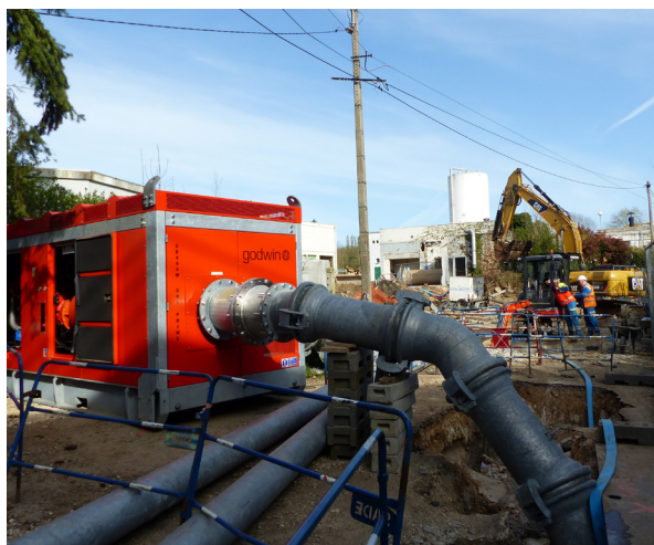
Xylem's Godwin pumps, equipped with Tier 4 engines, minimize air pollution by reducing the discharge of nitrogen oxide, as well as providing enhanced engine control and limited noise pollution
