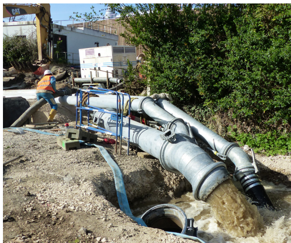
The existing sewer inlet at Lèves is connected to the bypass system as the wastewater is transferred to Mainvilliers
