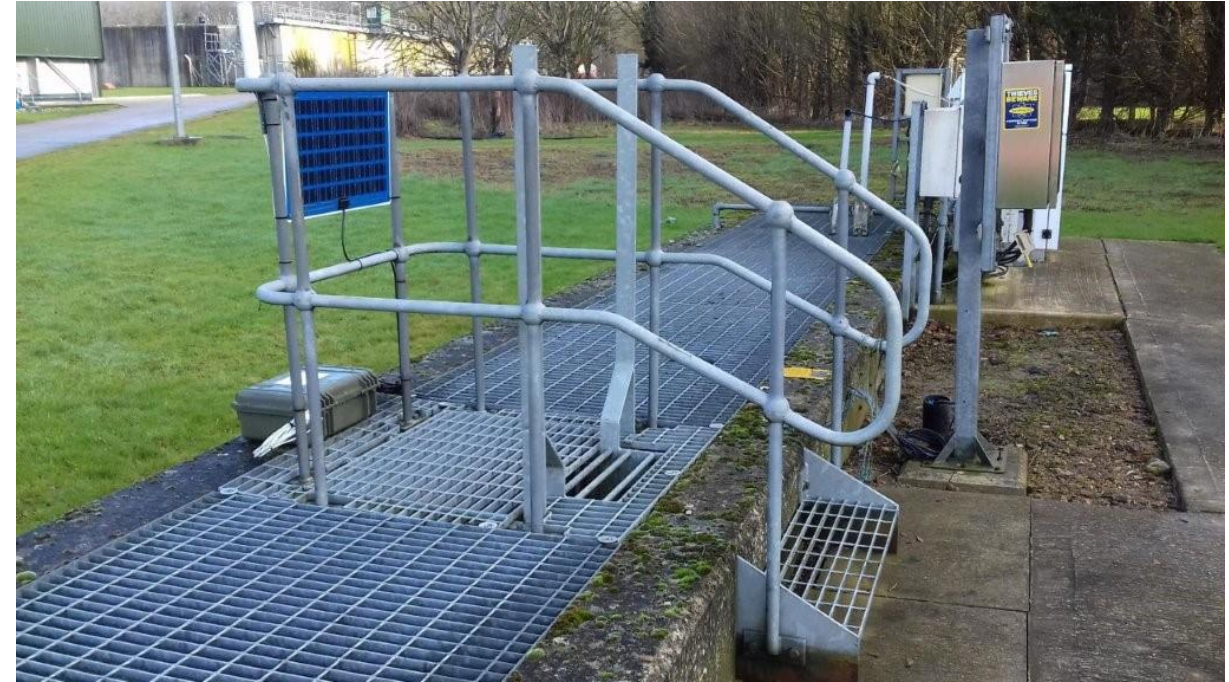
Final Effluent Monitoring in-situ to Cloud
