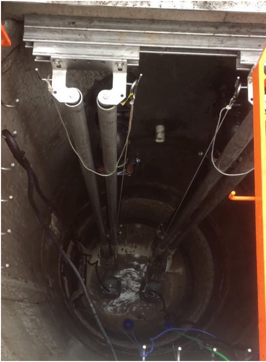
The Concertor XPC performing a wet well cleaning cycle to remove any debris from the pump station.
