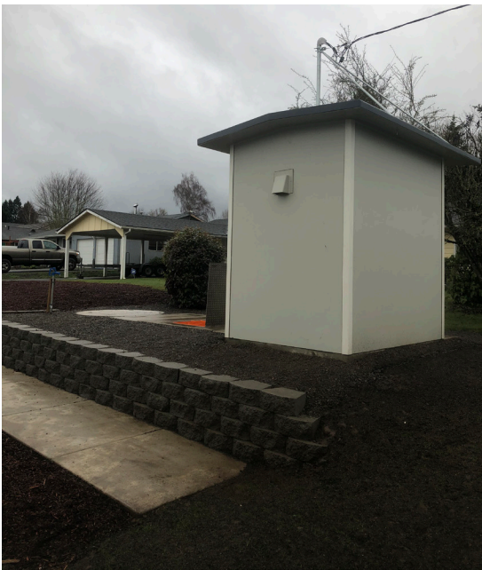
Concertor XPC pump station fully installed, complete with TOPS insert and new controls building.
