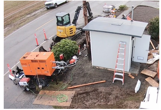
Godwin dewatering pumps ensuring continuity of operations during the installation of the new Concertor XPC pump station.
