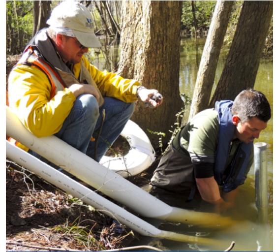
YSI field technicians installing protective casings for an EXO water quality sonde and discrete water sampler suction line.
