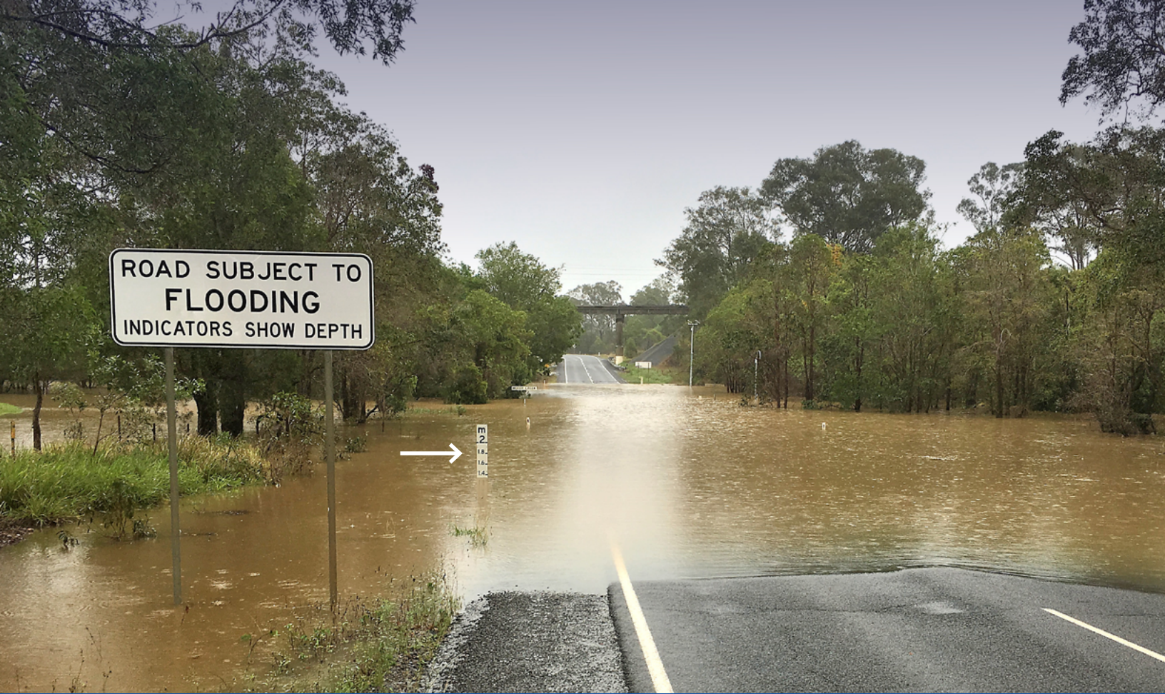
Road closure from flooding. Notice the staff gauge (arrow), a useful tool for drivers.
