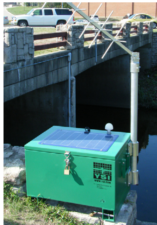
This portable water quality stormwater site in Kansas features a solar panel and is capable of collecting data, telemetry, water quality, MET, or flow in rugged applications.
