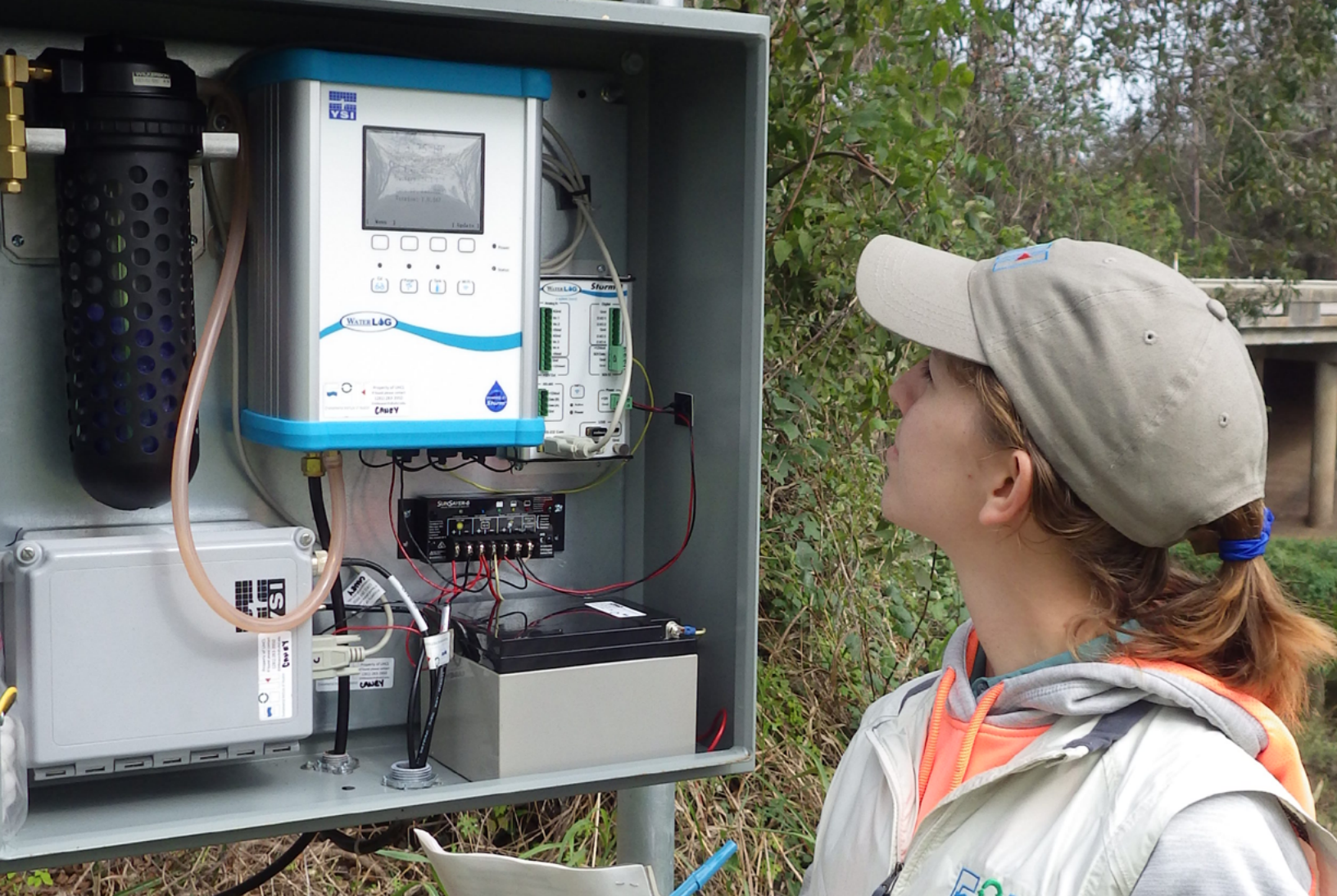
A complete stormwater solution featuring the Amazon Bubbler and WaterLOG Storm 3 Data Logger at a monitoring station in Texas.
