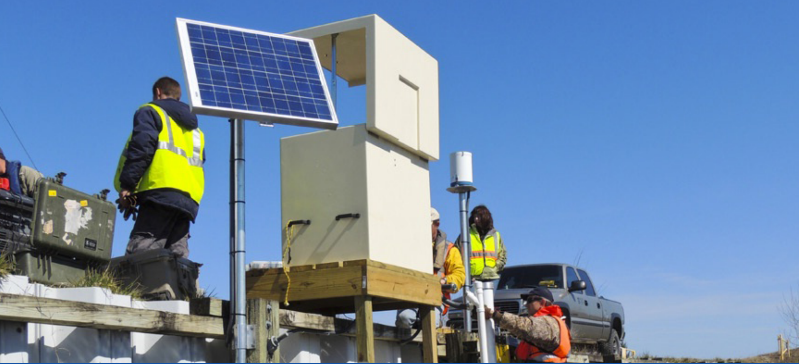
YSI's field services crew finalizing the installation of complete stormwater site in North Carolina.
