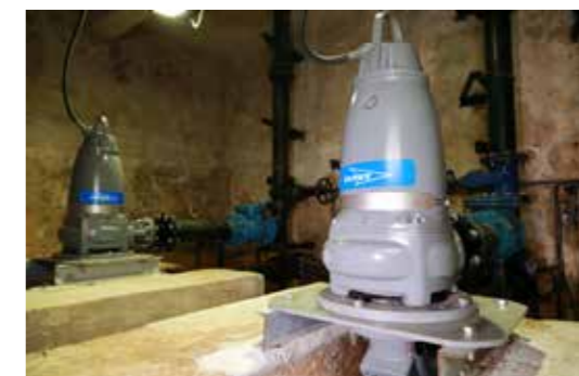
Flygt N pumps installed in pump station (dry installation).
