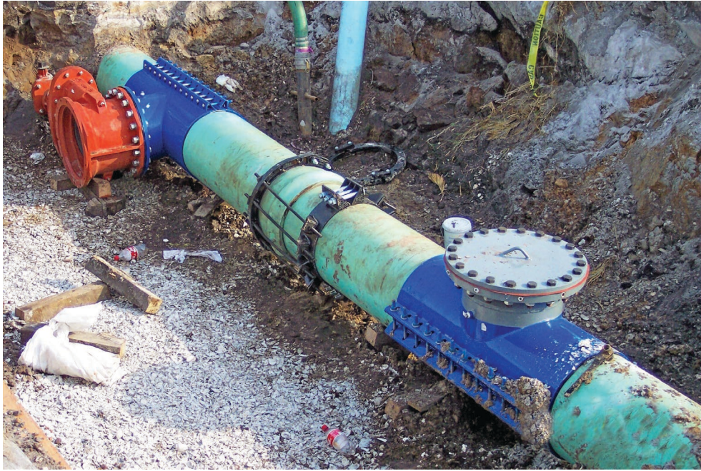
Line-Stop fittings installed in conjunction with tapping sleeves provide a means to isolate targeted pipeline sections without interrupting water service. Here we see a wastewater force main that will be relocated for a road widening project.
