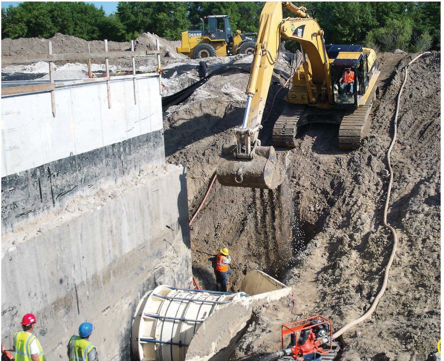
Trained Smith-Blair factory personnel are ready to assist with resolving the most complex on-site challenges.
