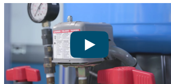
The 15 Typical Causes of Pressure Switch Chatter
