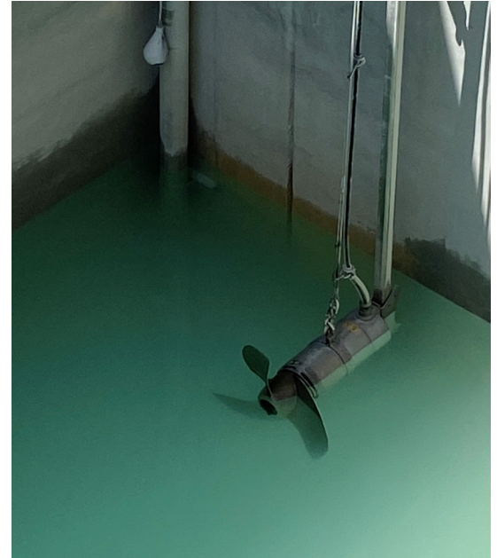
A Flygt adaptive mixer inside the tank.
